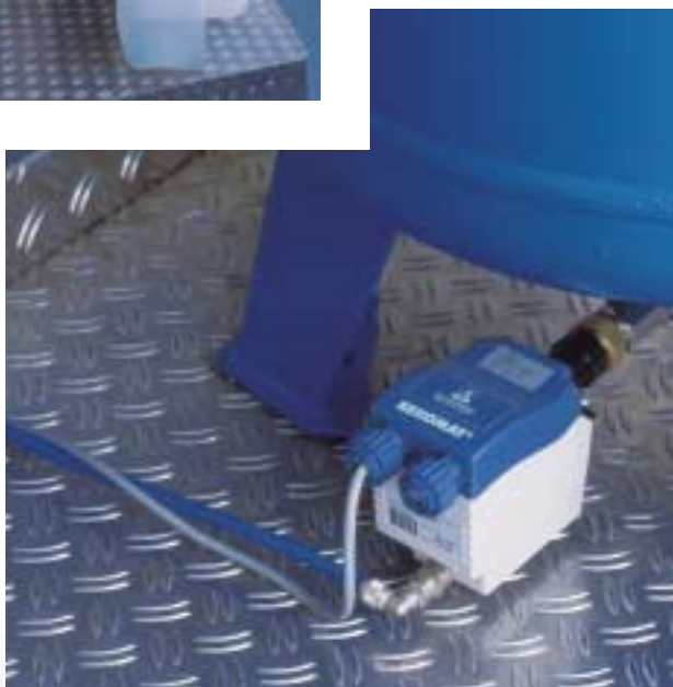
BEKOMAT® installed on air receiver
